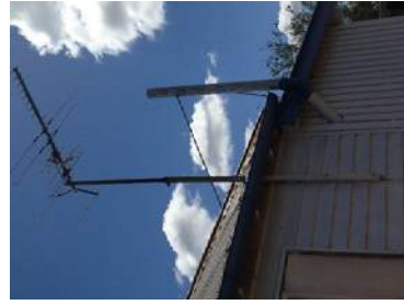
Existing TV aerial
